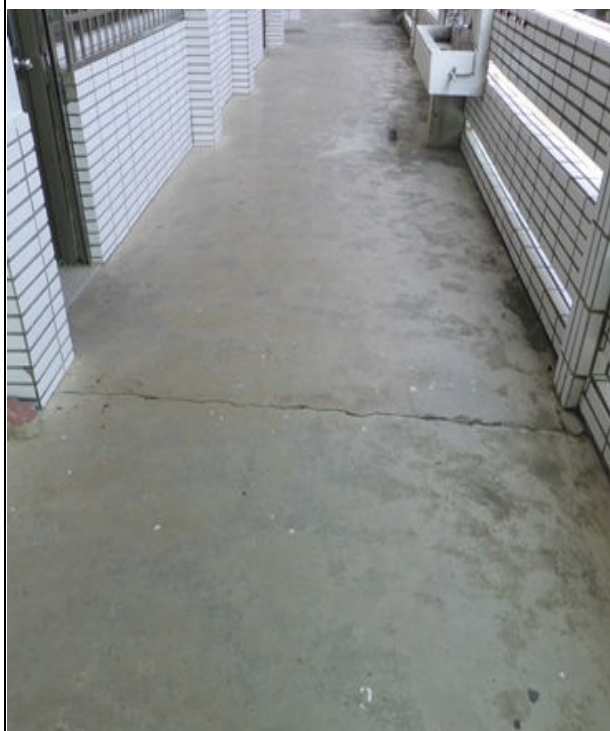
2樓底板貫穿式龜裂
